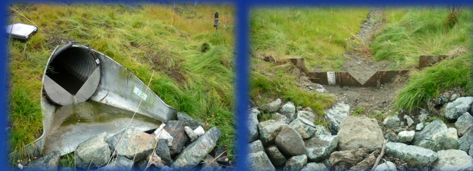
Basin inlet (left) and outlet (right)
